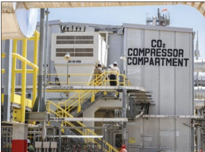
A CO 2 capturing plant in Hawiyah, KSA
