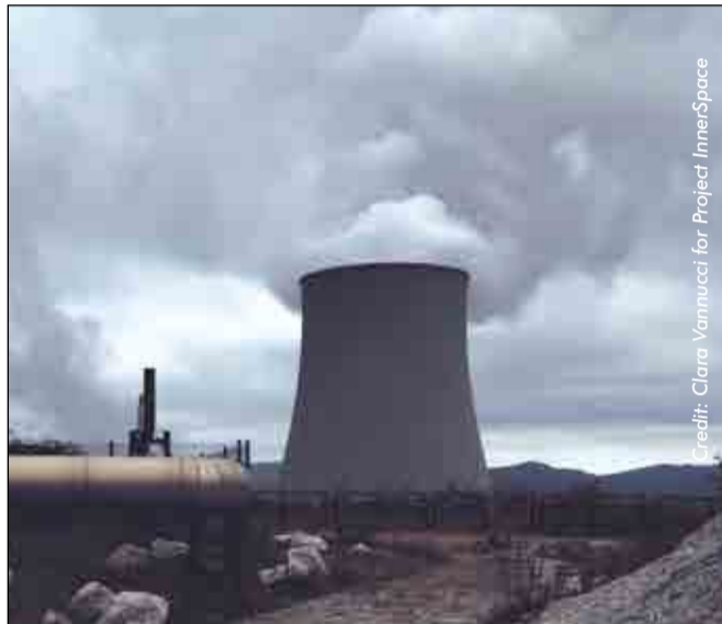
The Larderello Geothermal Energy plant in Italy ... the oldest geothermal plant in the world
