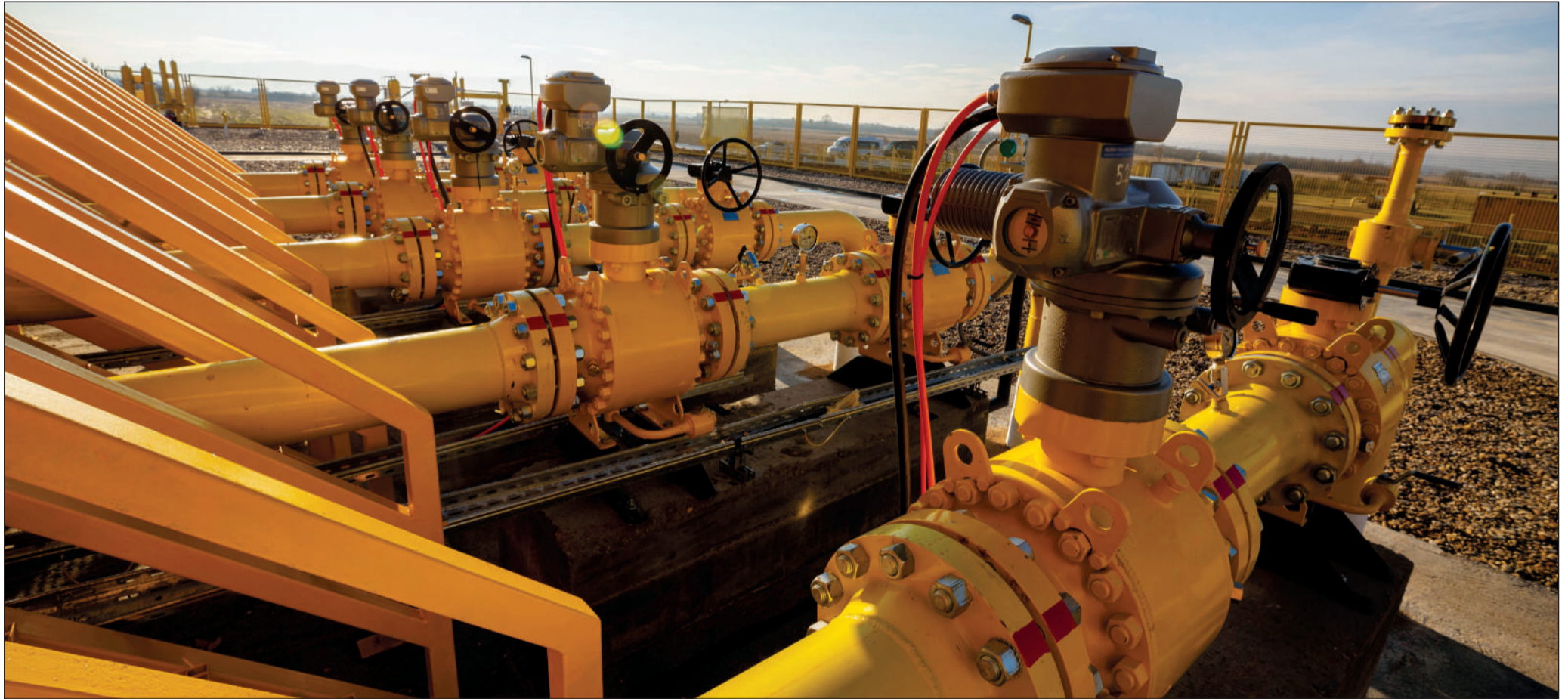
The construction of new loop lines aims to boost capacity and will aid OQ Gas Networks in meeting future gas demands
