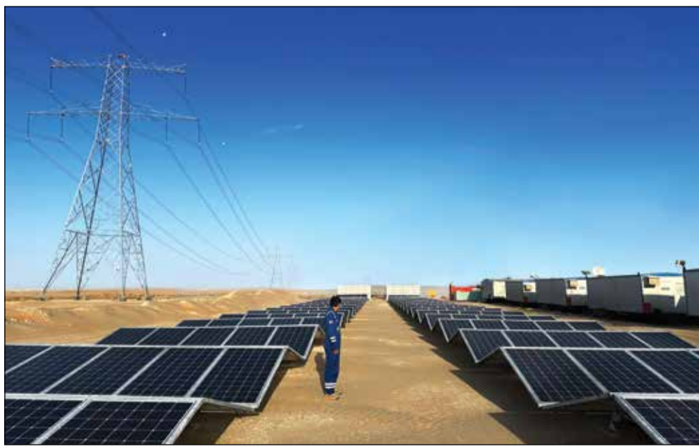
Mobile solar systems will replace generators for power supply
