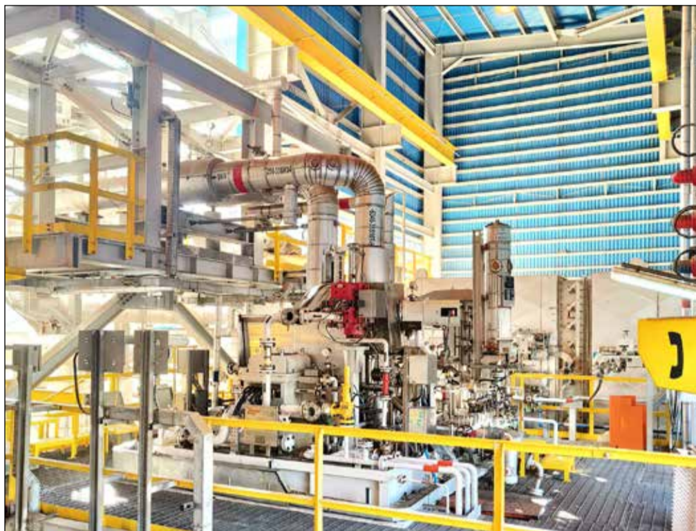
One of TTL's turbine generators for a Kuwaiti NOC
