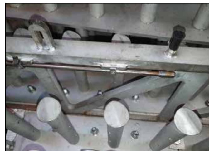
Sensors routing along internals
