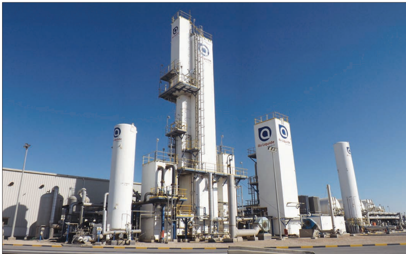
ALAR's hydrogen production site in Yanbu
